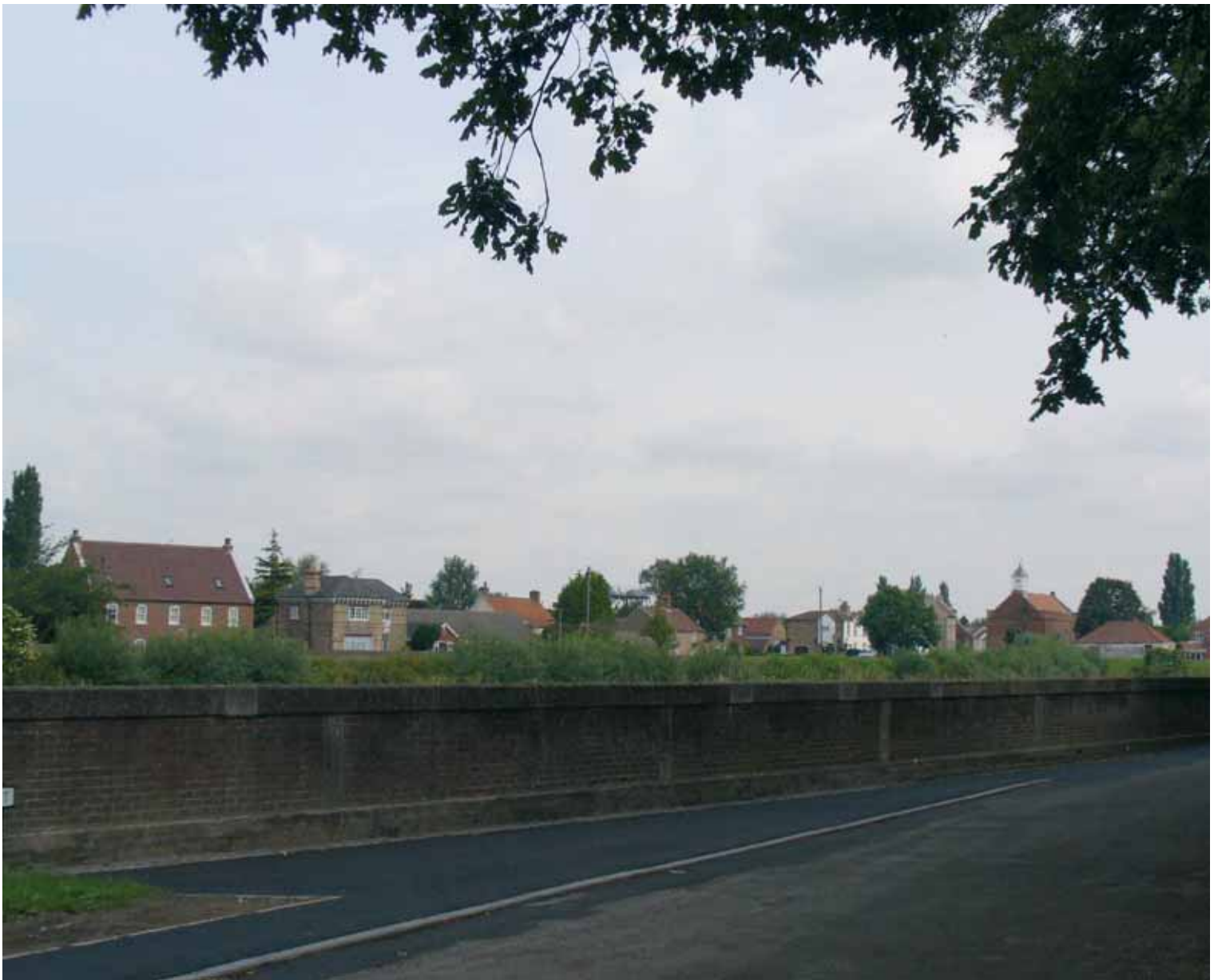
[6] View of West Stockwith across the River Trent interrupted by the flood bank constructed in poor quality materials
